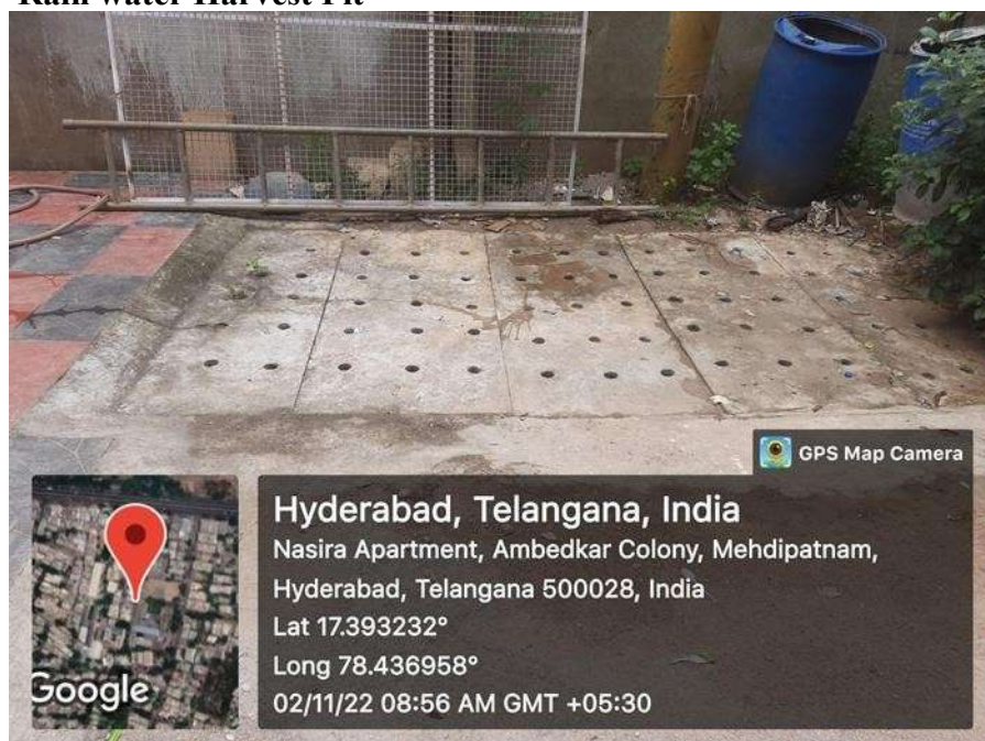
Rain water Harvest Pit
