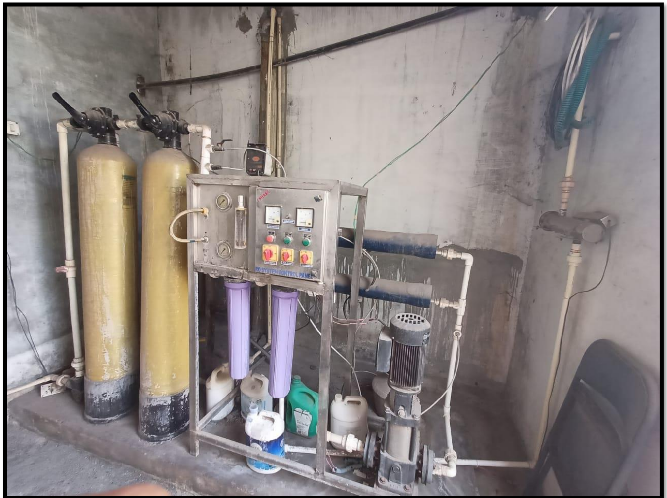
RO UNIT at St. Ann's
