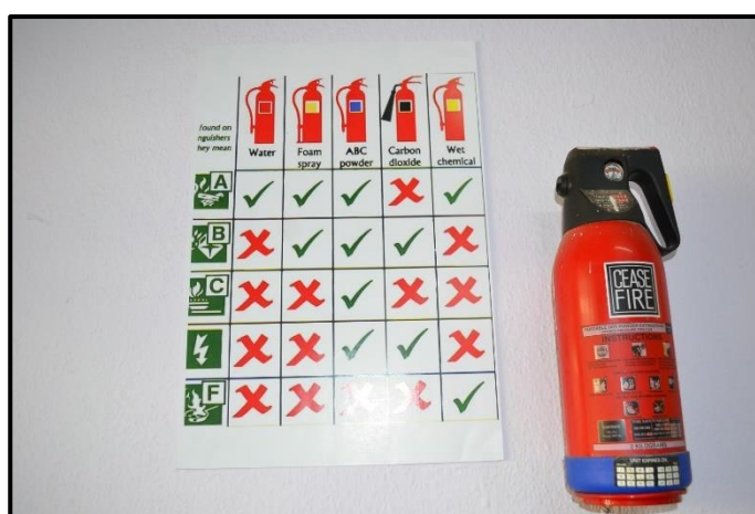
Safety measures in St. Ann's College for Women Campus
